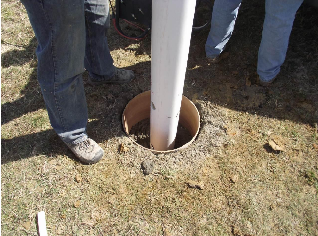
Figure 8. Position the PVC pipe at the desired location in the drill hole. Mark the PVC pipe at 2 ½ feet from the bottom. Insert the PVC pipe into the hole until the mark on the PVC pipe is at the same level as the top of the form.
