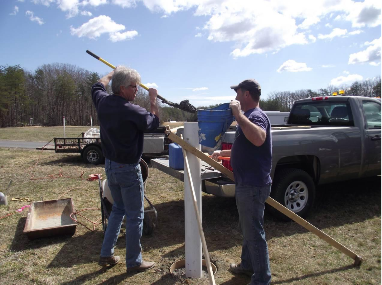
Figure 10. Fill the PVC pipe and form with remaining concrete. With the PVC pipe braced, fill the PVC pipe to the top with concrete. While adding the concrete into the PVC pipe, tap the sides of the pipe with a hammer to consolidate the concrete. Finish filling the form at ground level to the top with concrete, consolidate with existing concrete, and finish off the top surface.
