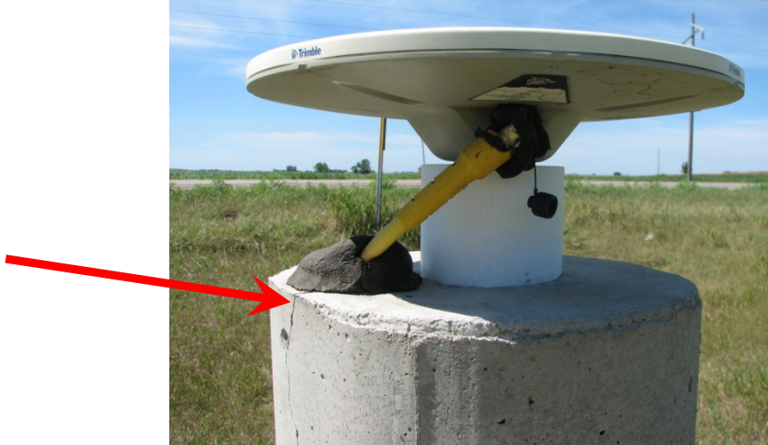
Figure 5 – view of pillar monument (note the crack that has developed near conduit location)
