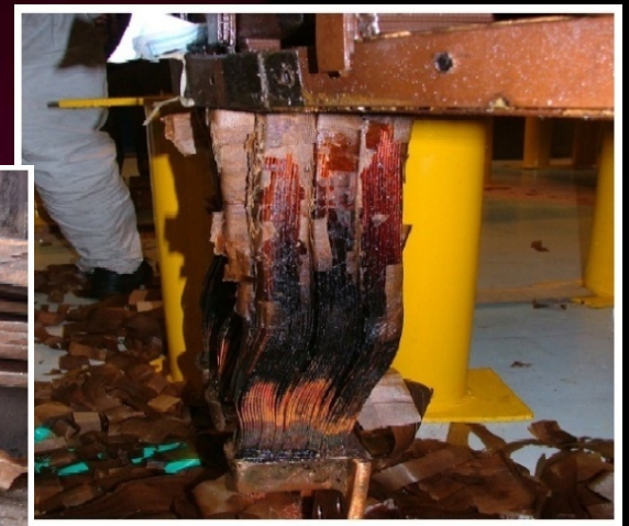
Transformer exit-lead overheating
