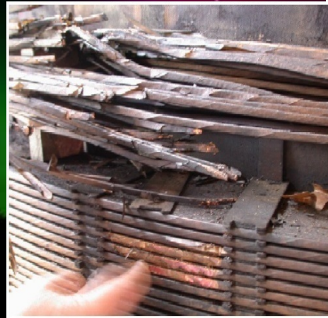
Transformer winding failure
